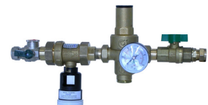
CA15C296PRV - Filling valve assembly comprising of – inlet Servicing Valve (AFL) c/w serviceable strainer, CA Device, Pressure Reducing Valve (PRV) and Servicing (isolating) Valve. Normally set to 1.5 bar
